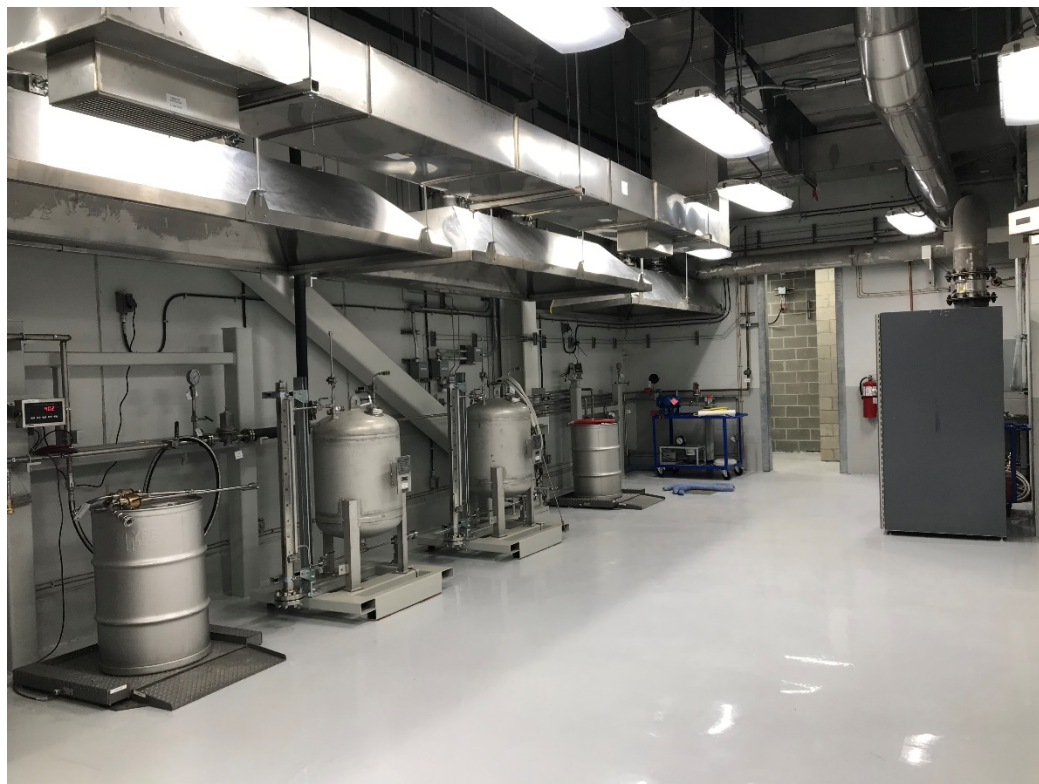
Figure 9 – Drum Handling, Cleaning and Testing Room
