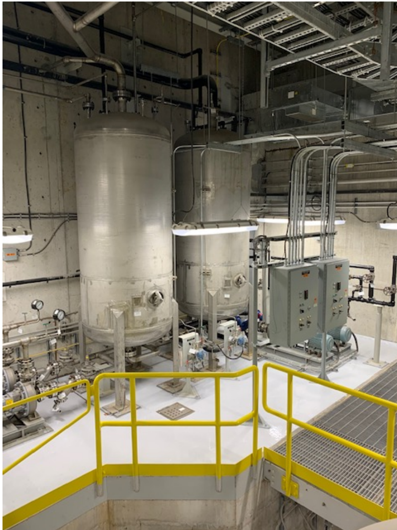
Figure 5 – Active and Inactive Drainage Tanks at Elevation 94 m
